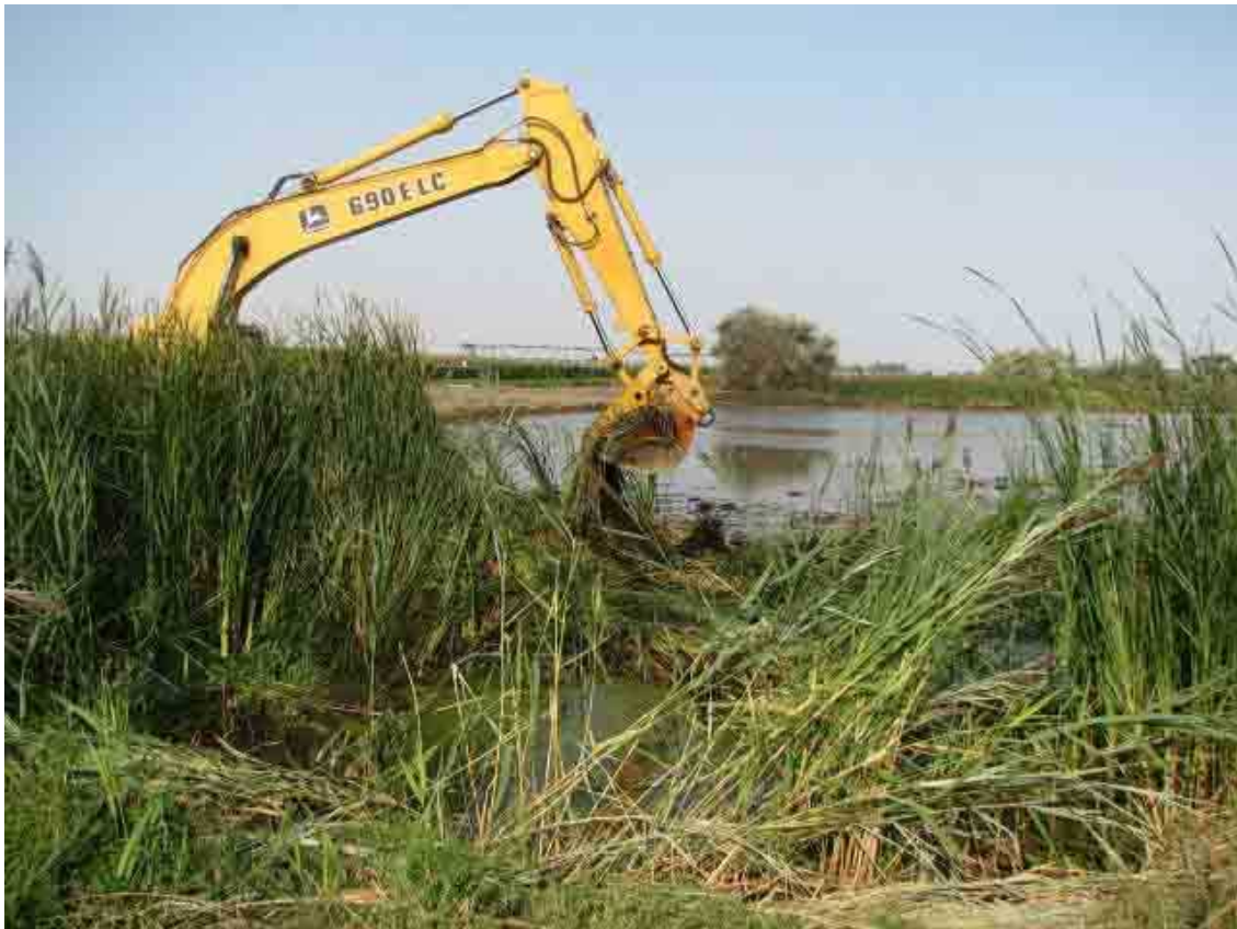
Heavy-duty equipment is used to tear out invasive phragmites weed that had choked off twenty acres of pond surface at McNary NWR
